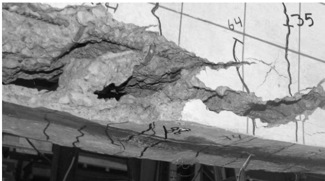
Figure 7. Concrete cover splitting failure
