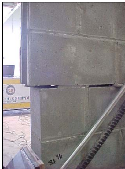
Fig. 3.5.3.1e Shear Sliding Failure
