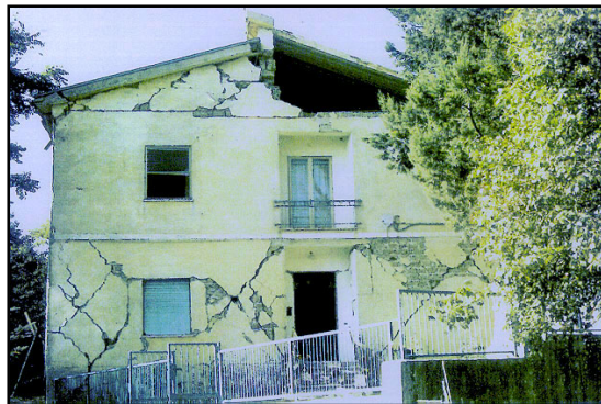
Fig.1.1.1c In-plane failure of load-bearing walls Umbria, Italy, September 1997
