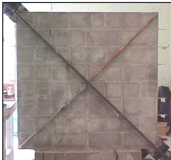
Fig. 3.5.3.1g Strengthened wall after failure
