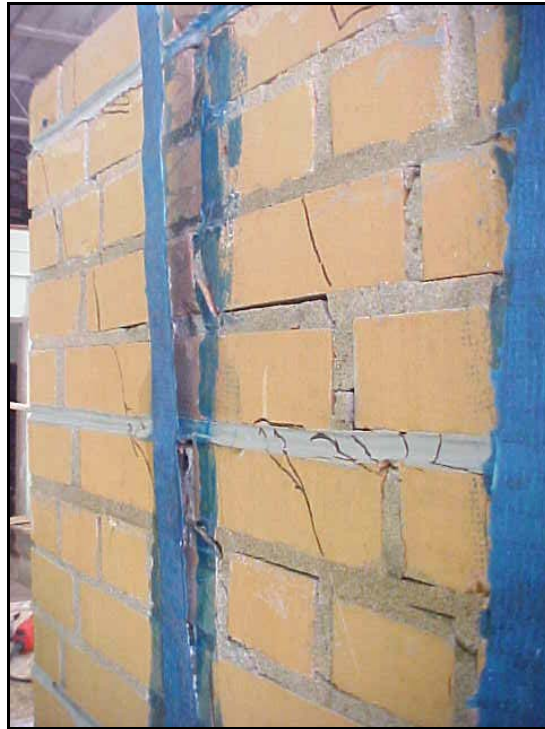
Fig. 3.5.3.2d Delamination of GFRP laminates from clay surface
