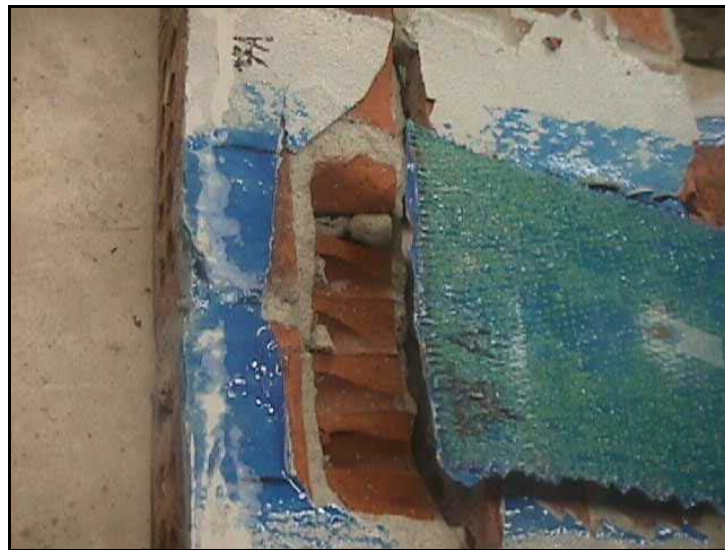
Fig. 2.3.5f*** Debonded laminate at the edge after failure
