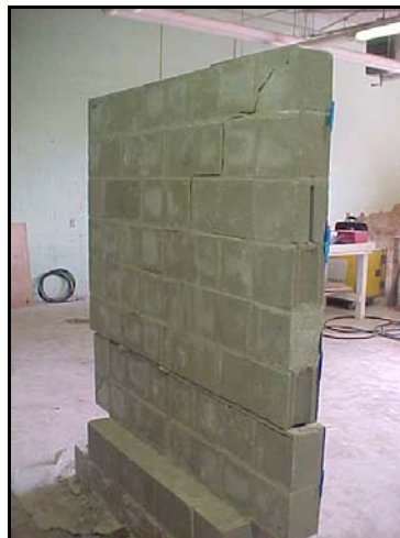
Fig. 3.5.1j Unstrengthened side after failure
