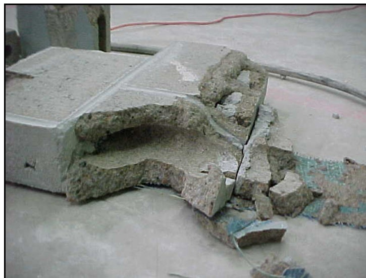
Fig. 2.3.5f* 45° fractures in concrete units
