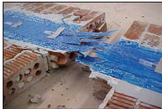
Fig. 2.3.5h*** Rupture of the GFRP laminate
