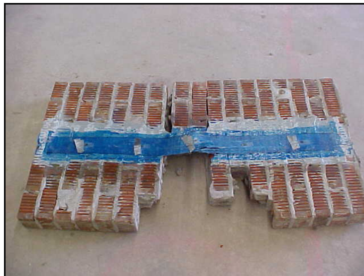
Fig. 2.3.5d** Rupture of GFRP laminate at mid-height
