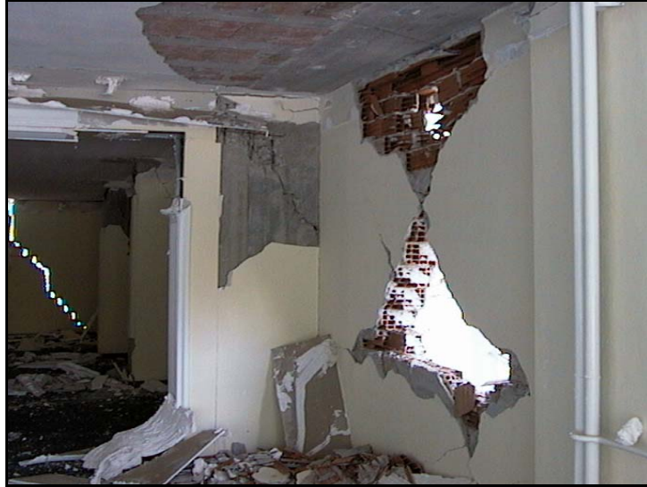
Fig. 3.1b Diagonal tension failure (Turkey 1999)
